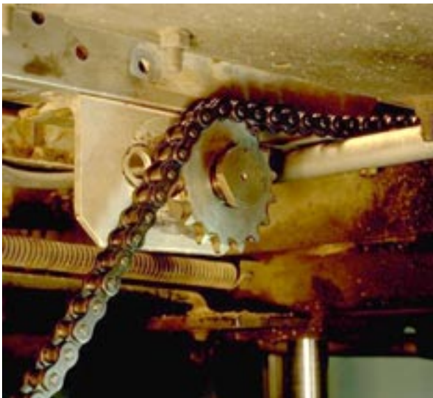
MT19 chain path showing chain slack, which can lead to brake shaft wear and failure.
